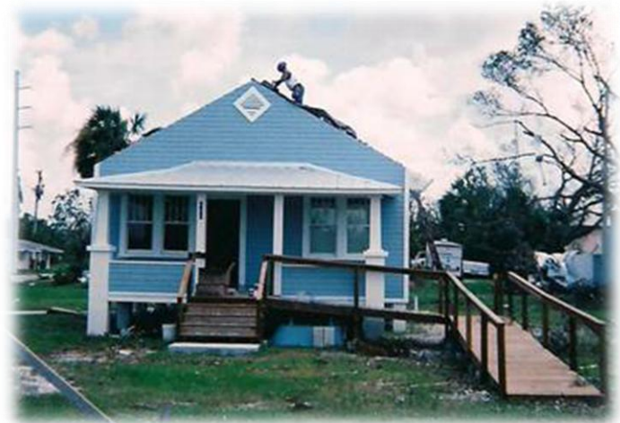
Hurricane Charley damage 2004
